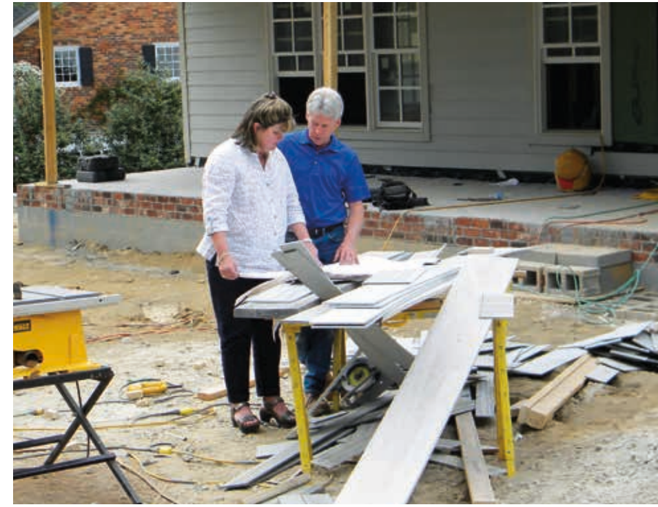
June Delugas and Don Hamrick review plans for the new home in Buena Vista.
